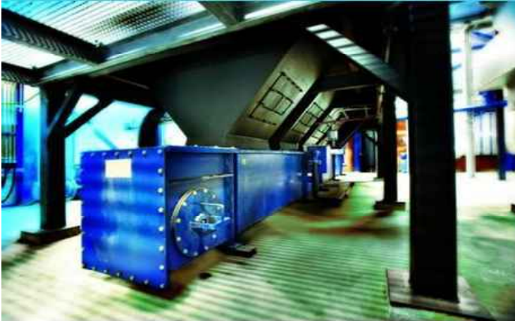
Figure 3.3: Wet ash conveyor
