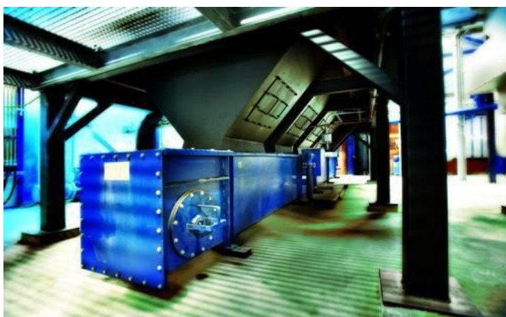
Figure 5.3: Wet ash conveyor
