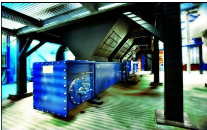
Figure 4.2: Example of Wet ash conveyor
