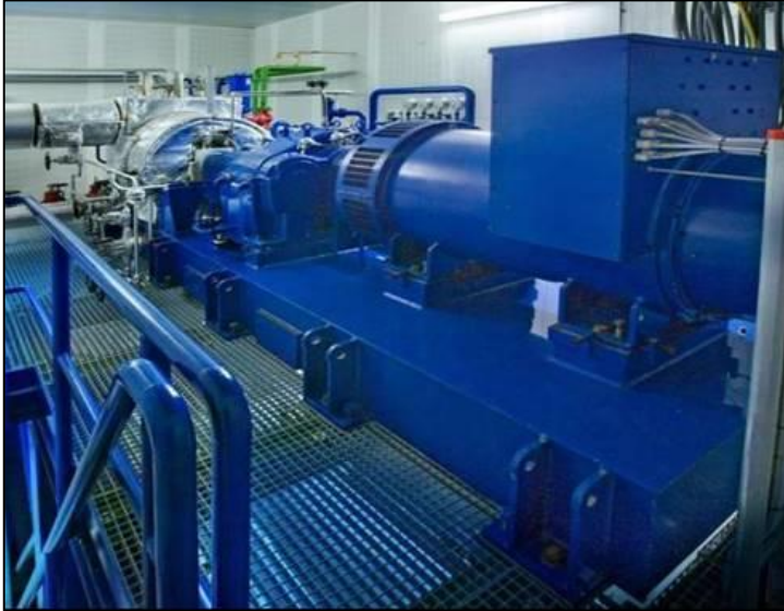
Figure 4.3: Example of Steam turbine
